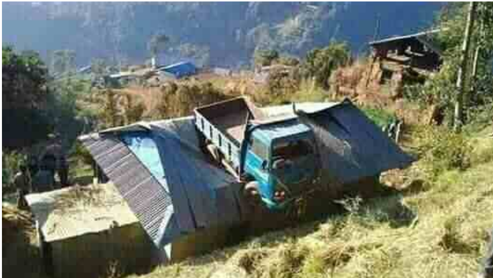
Figure 4: Roof was damaged but not the earthbag walls by this truck accident (C. Ziegler, used by permission).
