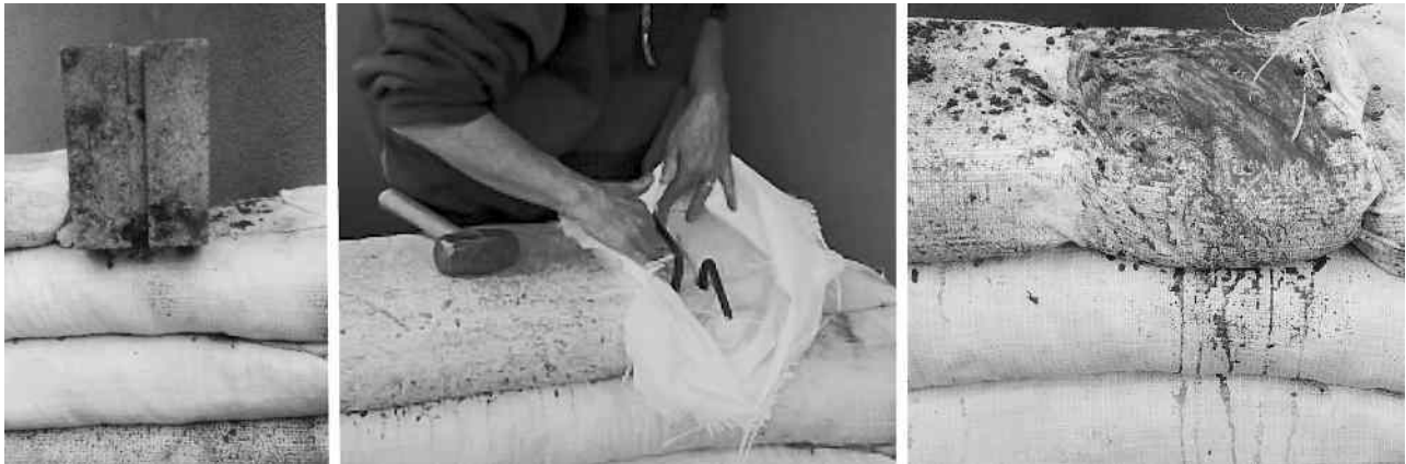
Figure 21 Open splice on current course (left to right): a- Tamp against a block to form gap; b- Insert vertical and/ or diagonal rebars; c- Fill tube with concrete and tuck end under.
