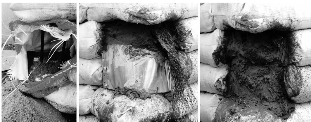
Figure 26 Making the splice (left to right): a- Remove sandbag fabric, b- Place form and use mesh to fill the top, c- Concrete splice with mesh trimmed.
