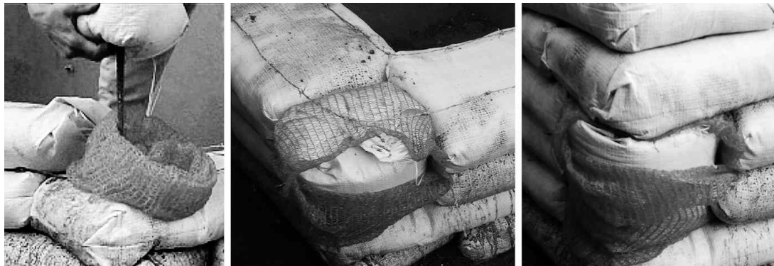
Figure 25 An upright sandbag for a covered splice (left to right): a- Insert the sandbag onto the rebar in the mesh; b- Build courses next to the sandbag; c- Build above splice to final wall height.
