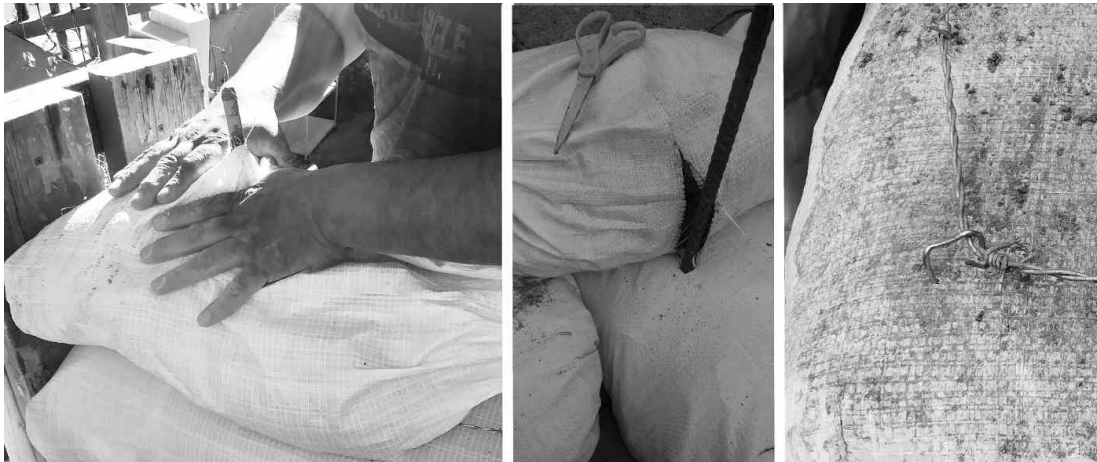
Figure 14 Better connections between steel and soil fill (left to right): a- Punch bags onto anchored rebar; b- Cut tubes to form around rebar; c- Tack wire corners taut with an electrician's staple.
