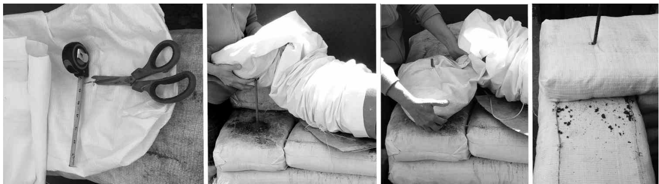
Figure 15 Punched-bag technique (left to right): a- Prepared hole near tube end; b- Slide a partly-filled tube end down over a rebar; c- Filled and tamped punched-bag with no fabric gapping.
