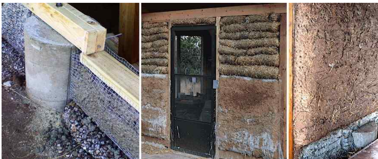
Figure 15 left: Gabion-type base wall between RC footings. Center: Panel of straw logs attached to studs with lower portion plastered. Right: Earth plaster leveling layers on interior of straw log infill panel.
