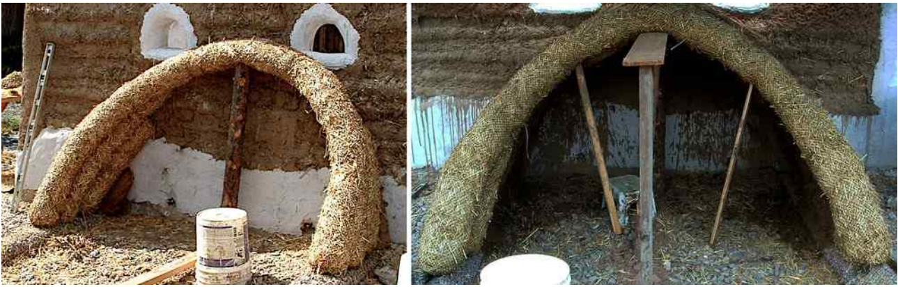
Figure 16: Left: Vault straw logs laid at slight angle against vertical wall. Right: Support for vault.
