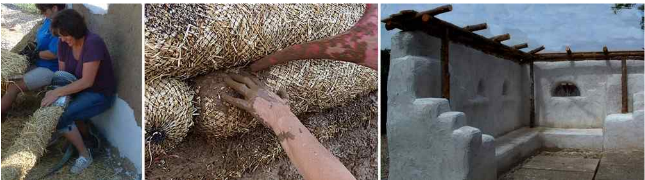
Figure 4 left: Stuffing straw logs. Center: Soaking logs with liquid clay. Right: Lime plastered straw log walls.
