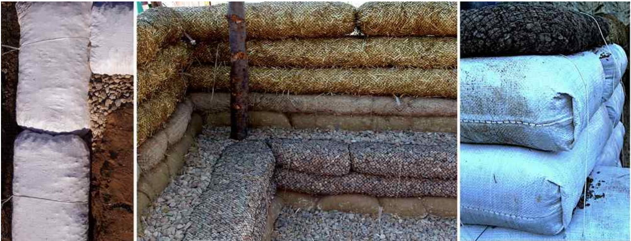
Figure 7 left: Gravel in bags for a water-resistant footing. Center: Gravel in wattle mesh makes a narrower course but is not damaged by water or by sun. Note that gravel bag below are coated with clay for temporary protection from sun. Right: Earth in wattle mesh on earthbag courses.
