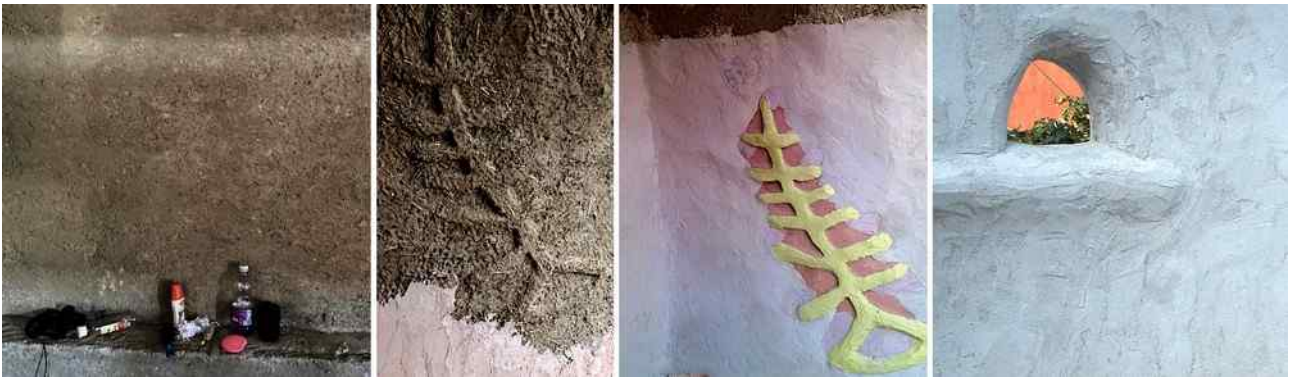
Figure 11 left: Stabilized earthen plaster forms a smooth Haitian dorm wall. Center: Straw-rich plaster forms raised designs on straw log walls, finished with colored lime plaster. Right: Lime plaster protects this LSC-shaped window sill from water on the straw log banco wall.
