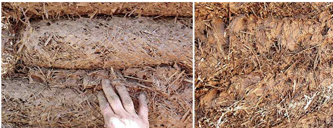
Figure 10 left: Push the first plaster firmly into the nooks. Right: Shaping plaster will stick more easily.
