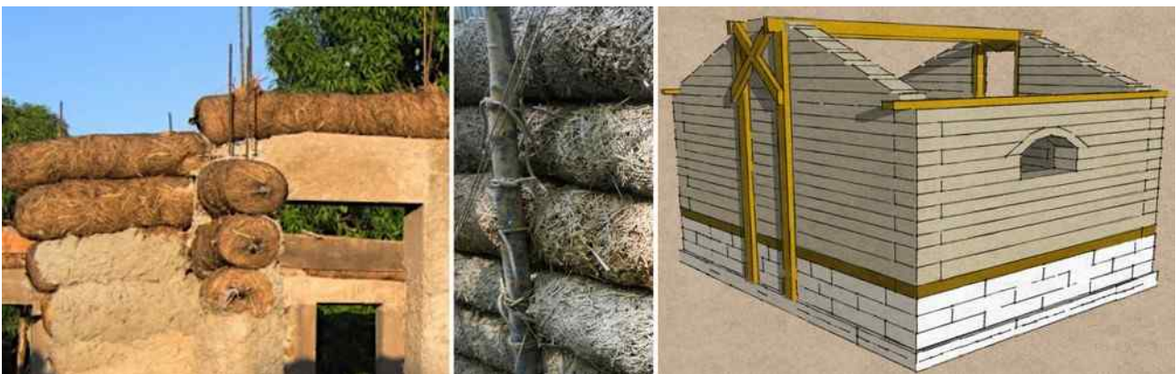
Figure 5 left: Haitian dormitory impaled oversized straw logs on rebar. Center: Poles can be tied into log mesh. Right: Small straw log shelter planned for wood posts attached to earthbag support roof beams.
