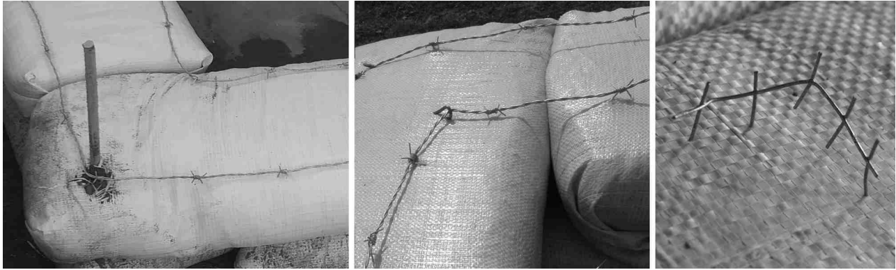
Figure 11 Hold barbed wire in place (left to right): a- Wrap around a vertical rebar; b- Tack wire at corners with an electrician's staple; d- Tack with pins cut from wire mesh.
