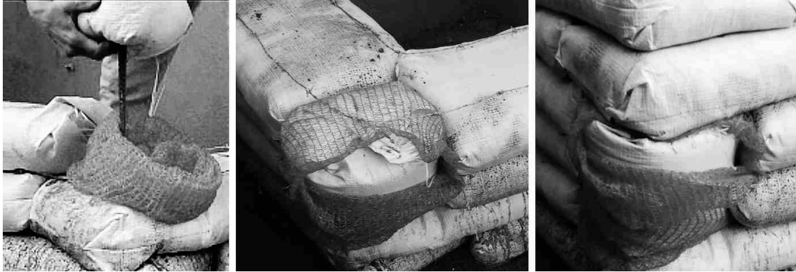
Figure 26 Covered splice preparation (left to right): a- target sandbag inserted over rebar into mesh tube; b- courses laid next to the sandbag; c- courses added above the sandbag.
