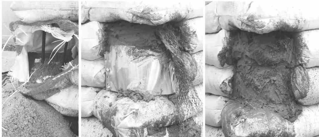
Figure 27 Casting a covered splice (left to right): a- Remove sand and sandbag fabric, b- Place form and use mesh to fill the top, c- Concrete splice with mesh trimmed.
