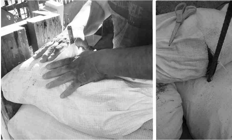
Figure 20 Rebar in walls (left to right): a- Punch bags onto anchored rebar; b- Cut tubes to form around rebar.
