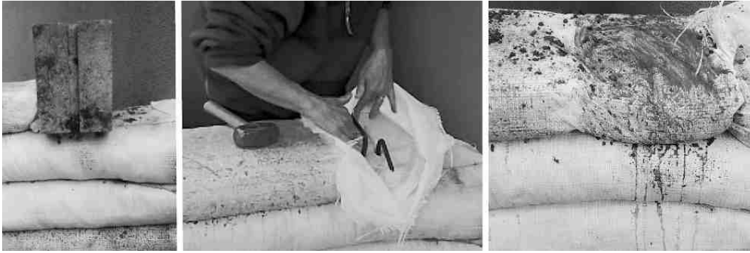
Figure 24 Splice on current course using tube as concrete form (left to right): a- Insert diagonal; b- Insert vertical; c- Both hooks fit within tube form on wall top.
