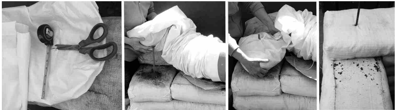
Figure 22 Punched-bag construction (left to right): a- Prepared hole near tube end; b- Slide partly-filled tube end over a rebar; c- Locate and firm the tube end; d- No fabric gapping after filled and tamped.
